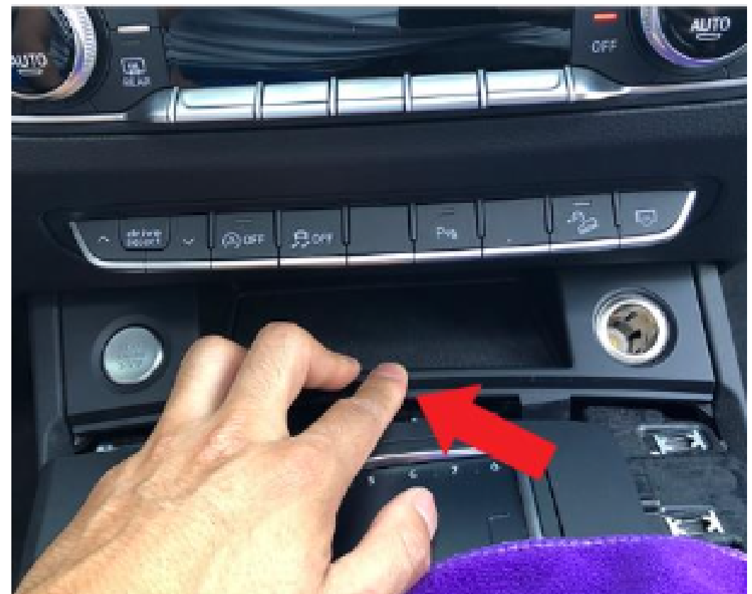
24. After properly installing the climate control trim, proceed to reassemble everything starting with the installation of the start button panel.
